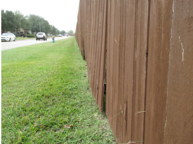
Loose and deflected pickets
