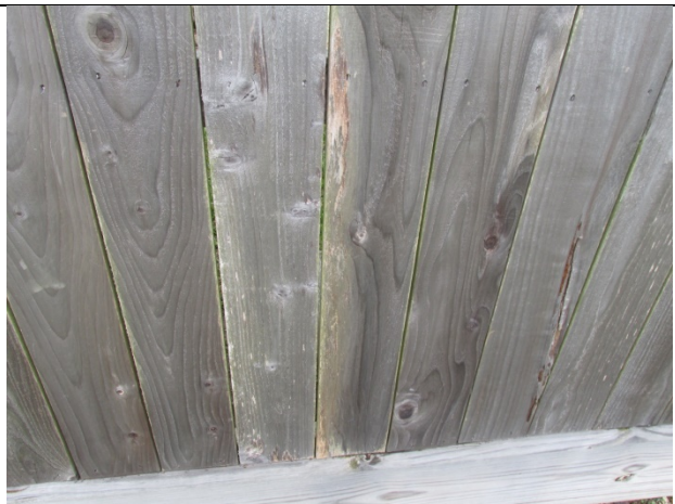
Wood deterioration at Miller Ranch Road
