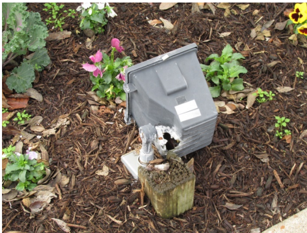
Damaged light fixture
