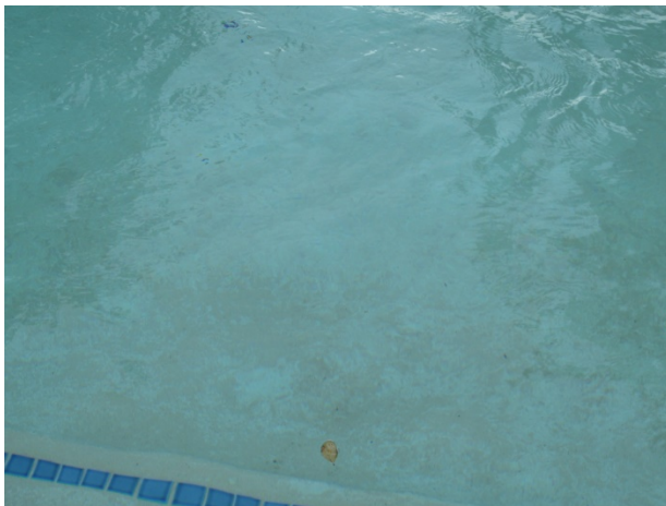
Plaster finish deterioration
