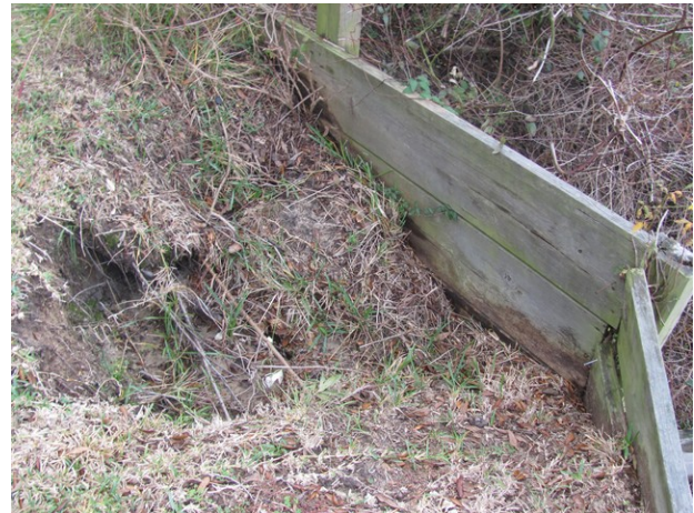
Erosion behind retaining wall
