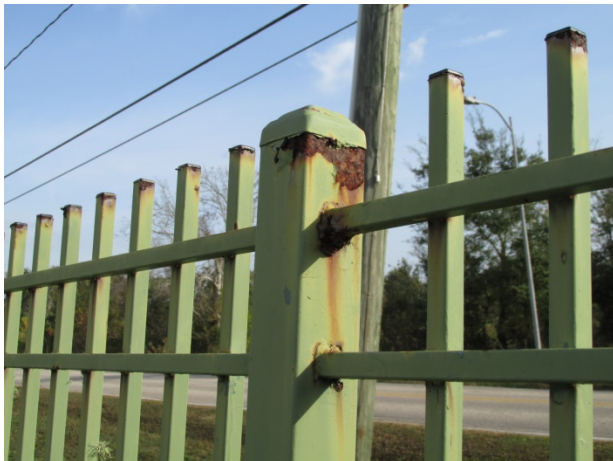
Finish deterioration and rust
