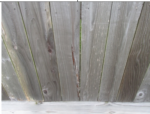
Wood rot at Miller Ranch Road
