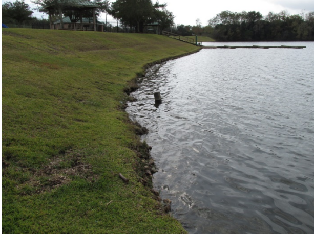
Minor shoreline erosion
