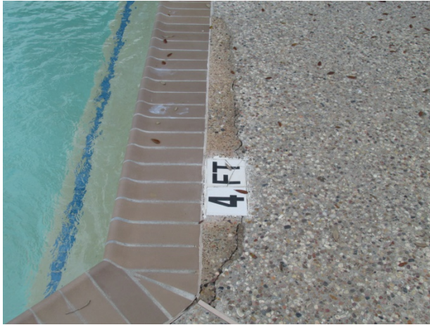
Concrete deck cracks
