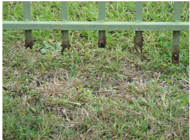
Rusted and deteriorated rails
