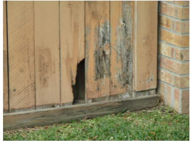
Finish deterioration and damage
