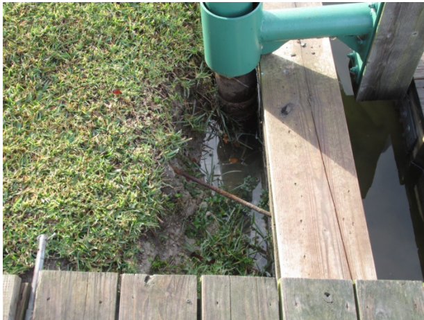
Shoreline erosion by bulkhead
