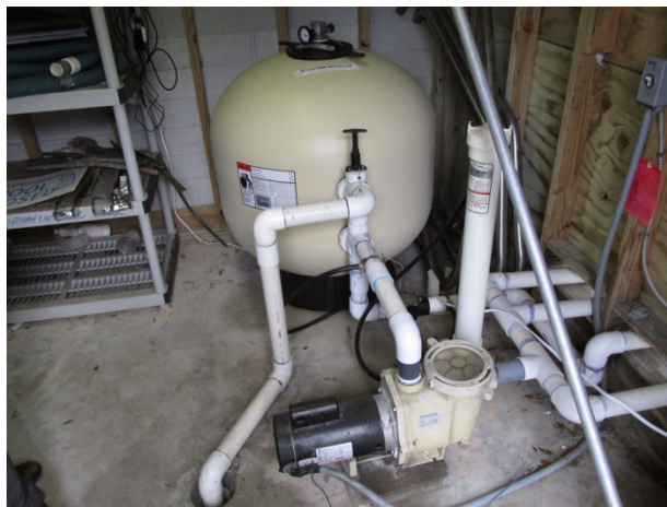
Pool mechanical equipment
