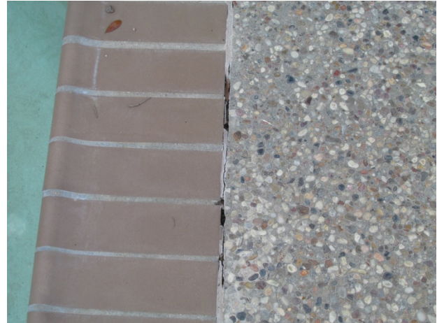
Sealant deterioration between pool coping and deck
